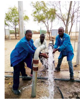
Solar powered borehole pumps at the Dagahaley refugee camp in Kenya
